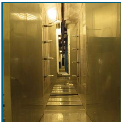
AR Powder Coating features an 8-gun automated painting station paired with a down-draft system.
